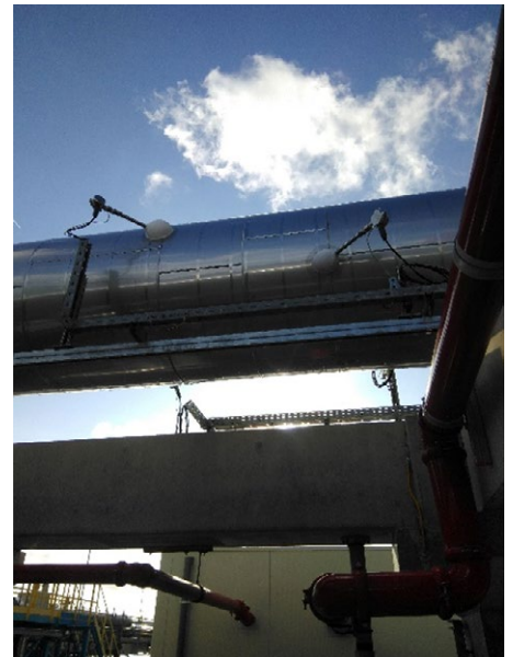
Fig. 2 and 3: LNG flowmeter with FWPA+BWT transducers
