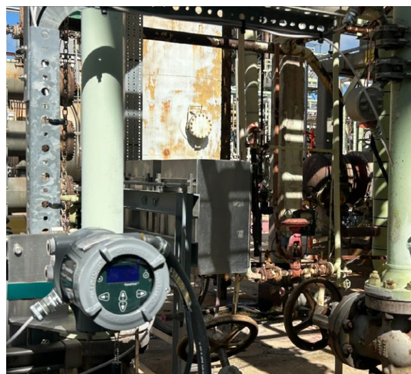
Fig. 1: PanaFlowLC installed in 2025 (with transducers at the top right)
