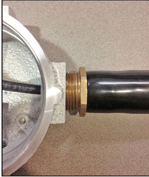
Figure 17: Torquing the Cable Gland
