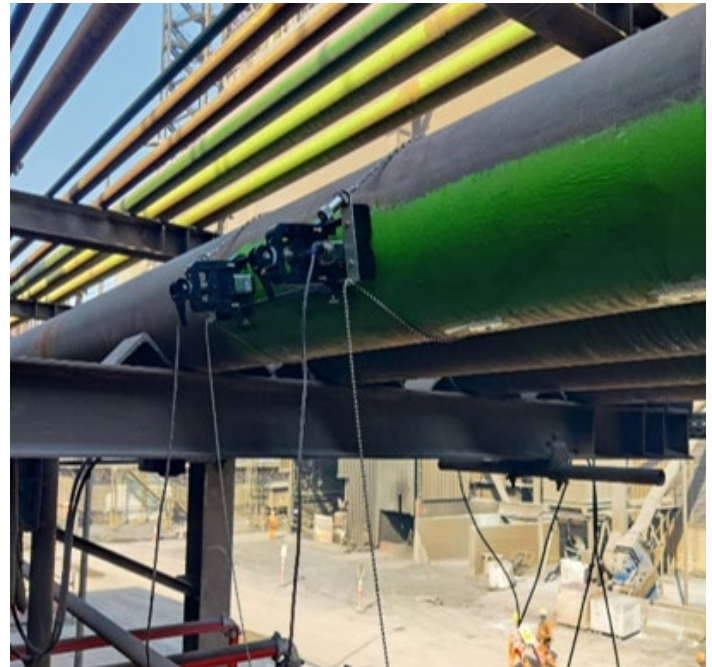
Pic. 1: C-RR 1Mhz on DN300 CS cooling water pipe
