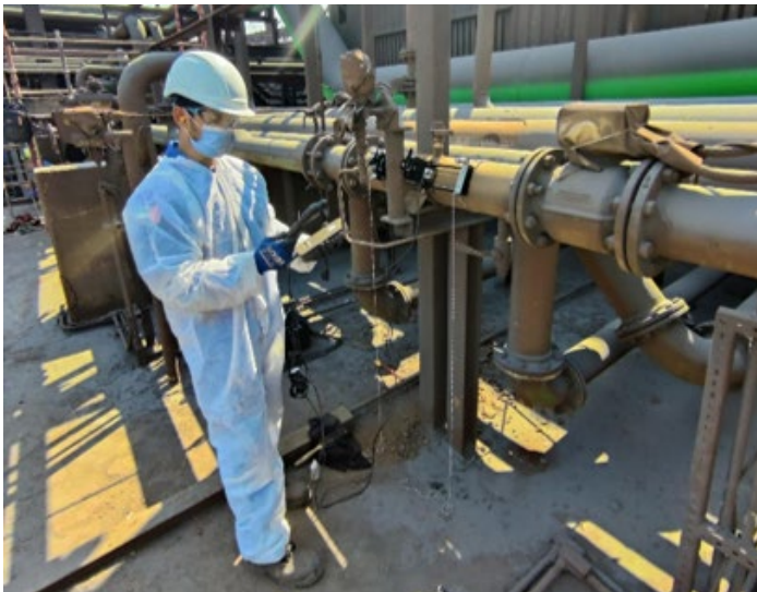
Pic. 3: PT900 installed to verify the existing Magnetic flowmeter
