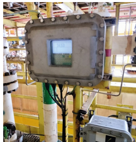
Fig. 1: Existing ultrasonic flowmeter
