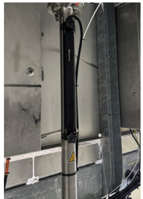
AT20 transducers installed on the cooling line
