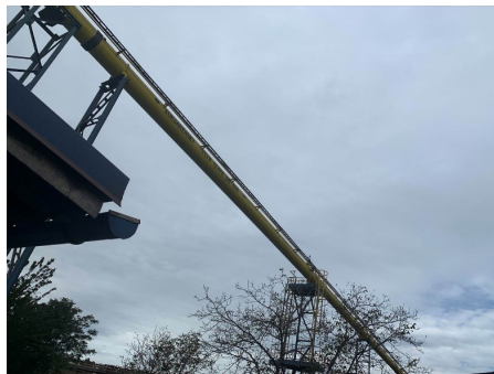
Picture 12. DN800 coke oven gas
