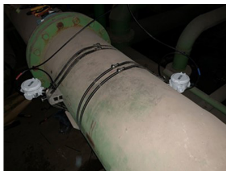
Picture 3. 50-year-old corroded pipe
