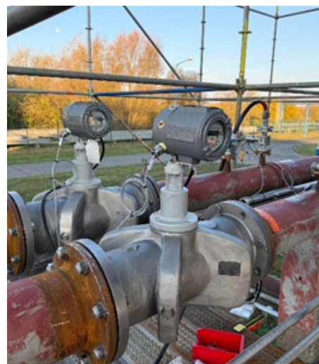
PanaFlow ZIG installed on the gas lines
