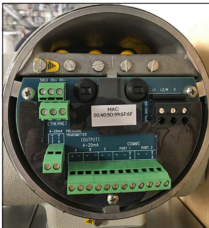
Figure 25: Wiring Terminal Blocks
