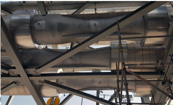
Fig. 2: Former Venturi Flow meter
