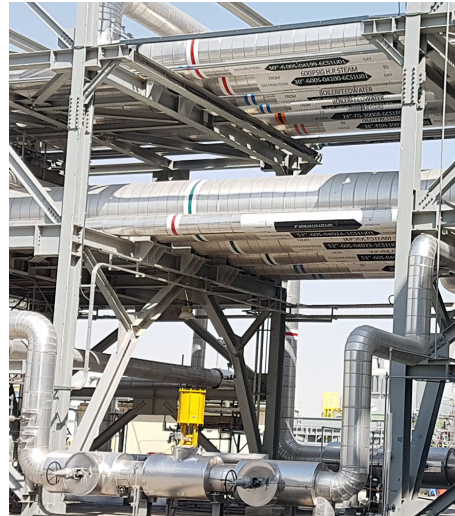
Fig. 3: Insulated steam line
