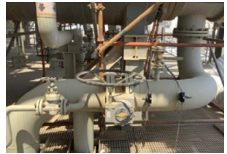
Fig. 2: Cooling water inlet of one heat exchanger with no straight runs
