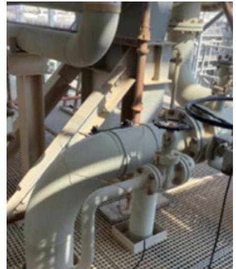
Fig. 3: Cooling water inlet from another heat exchanger with no straight runs
