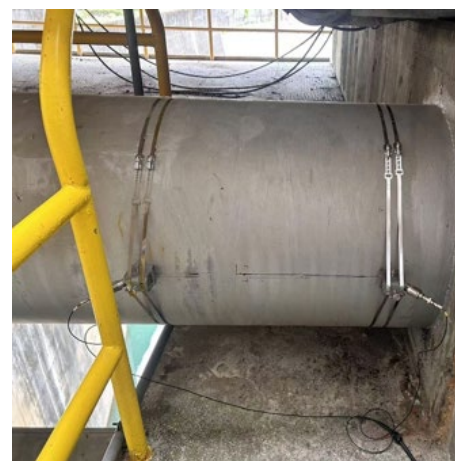
Fig. 1: C-RS 0.5MHz installed on DN700 pipe
