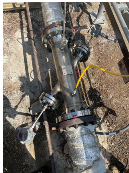
Panametrics ultrasonic steam flowmeter
