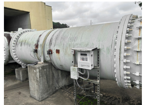
Existing DF868 with C-RS 401 on another influent wastewater line
