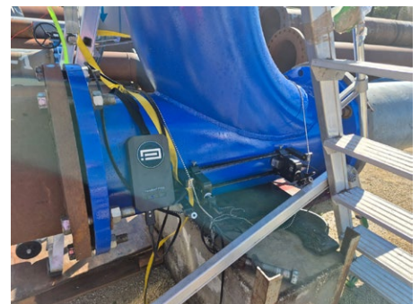
Fig. 1: PT900 attached to robot insertion mechanism (DN400)
