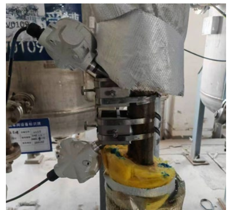
Fig. 1: C-PT 1 MHz installed on 2" SS line
