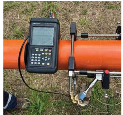
Fig. 2: PT878GC installed on the main 6" CS line
