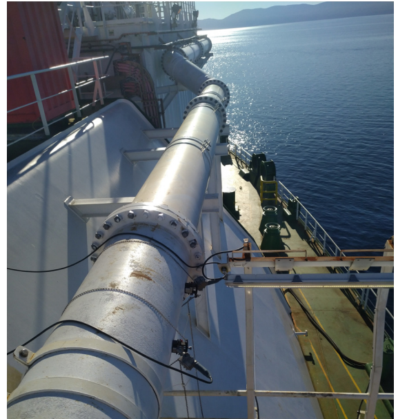
C-ET transducers installed on the heating water line
