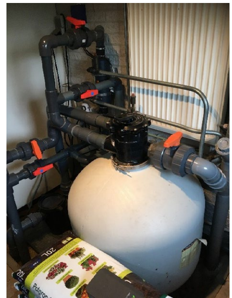
The complete filter installation
