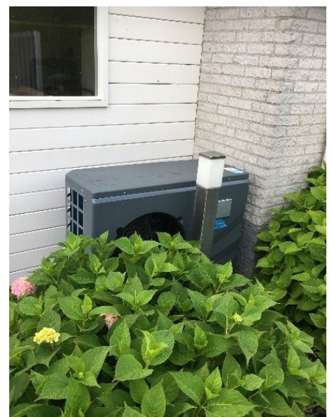
The 20kW heat exchanger
